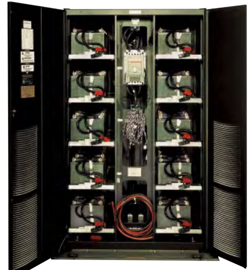
IBC-L with doors opened
